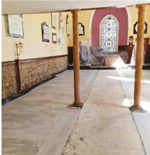
The new floor in St. Sillian's Church supported by the Benefact Trust.
