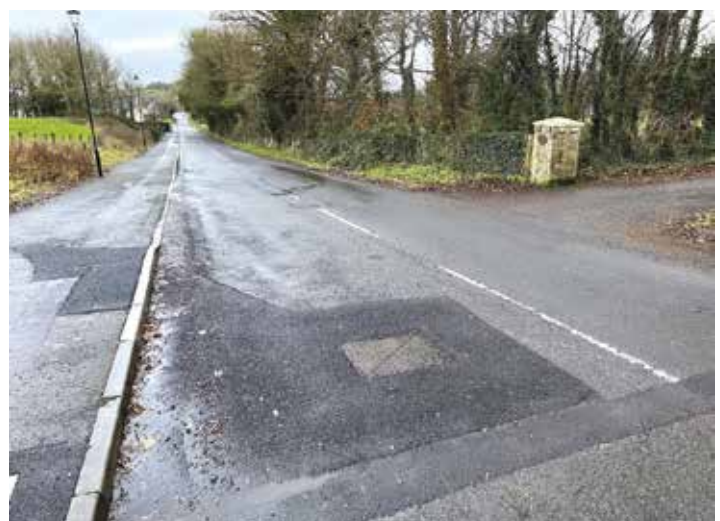
Photo shows the position of the defect in the foreground, with Waterhen Lane travelling down towards the River Erne.
