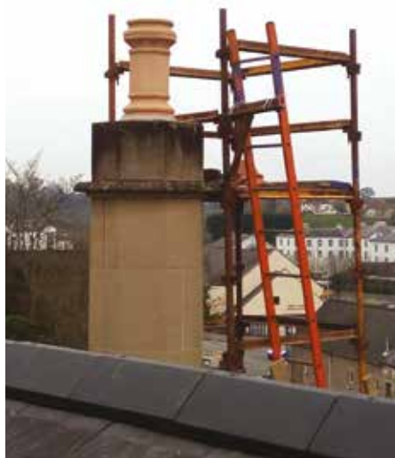
Other work undertaken to secure the building into the future included the replacement of the old chimney pot which had deteriorated as a result of frost damage.
