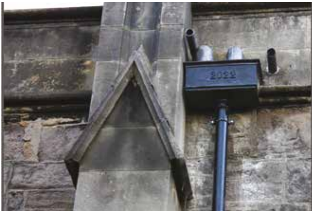
The new cast iron hopper, with the 400th anniversary date, which takes the roof water from the centre section of the roof over the south aisle.
