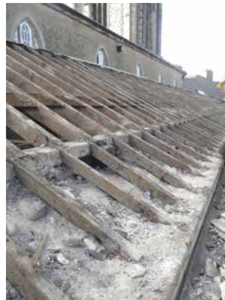
The rafters on the north side of roof showed signs of decay, especially those end pieces in contact with the wall.
