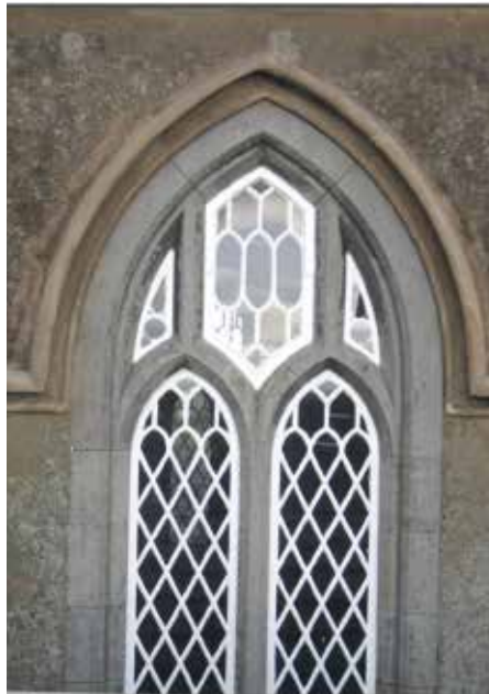
A restored and freshly painted high level window. Plaster work on the high-level windows required repair, due to age and weather damage.
