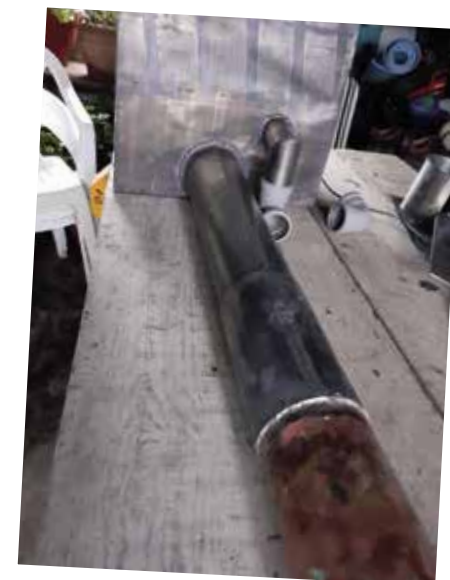
The completed lead sump with the outflow pipe. Note the small diameter overflow pipe which will give prior warning of any build-up of debris in the sumps.
