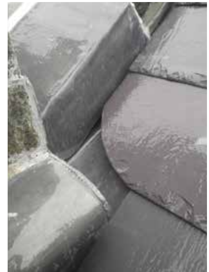
The picture shows new lead which has been carefully crafted at the base of a roof pinnacle.
