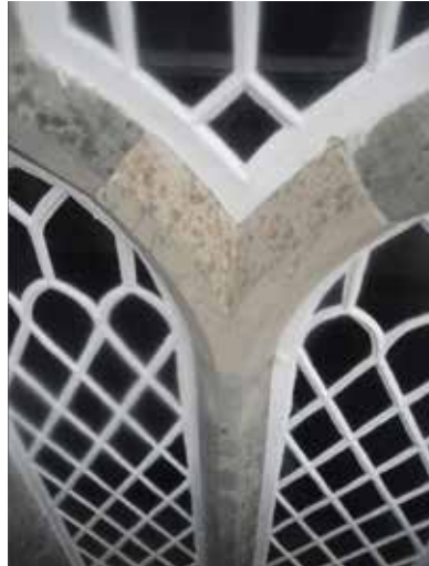
The picture shows a section of a high-level window surround which has been replaced in an impressive manner.
