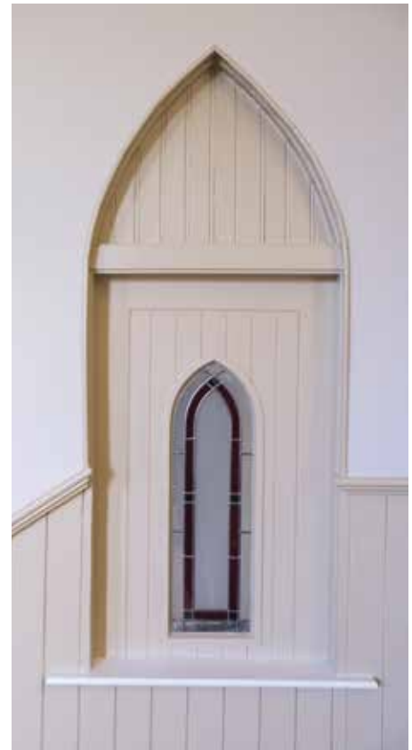
An interesting feature in the new refurbishment is this arch where a door was once fitted.
