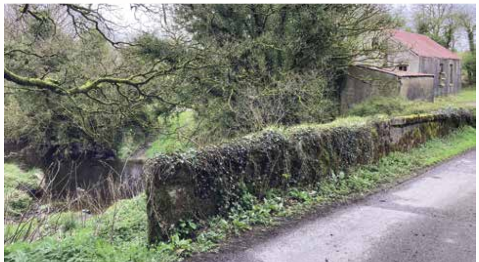
The bridge over the Termon River with the former Termon Creamery premises in the background.
